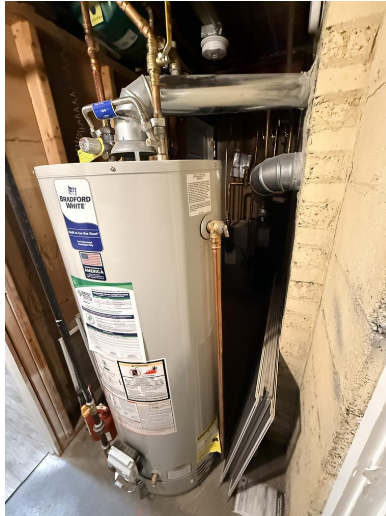
Figure 59: Basement, Hot Water Tank
