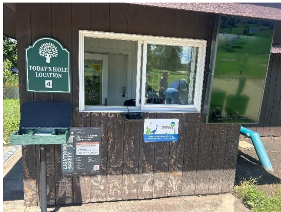
Our 9-hole starter hut was showing severe signs of wear-and-tear.
