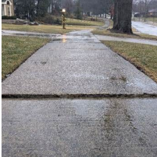
_____ Trip Hazards (e.g. uneven sidewalk panels)
