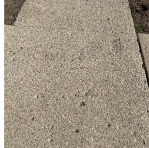
_____ Poor Surface Quality (e.g. broken sidewalks)
