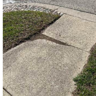
_____ Standing Water/ Debris (e.g. standing water, ice)
