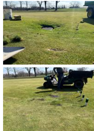
Top picture shows a sunken drainage collection area on hole 7. Bottom picture is the same area after the repair.
