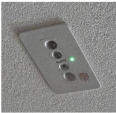
Emergency lights were replaced throughout R22. Bottom picture is of our new low profile more modern light fixture
