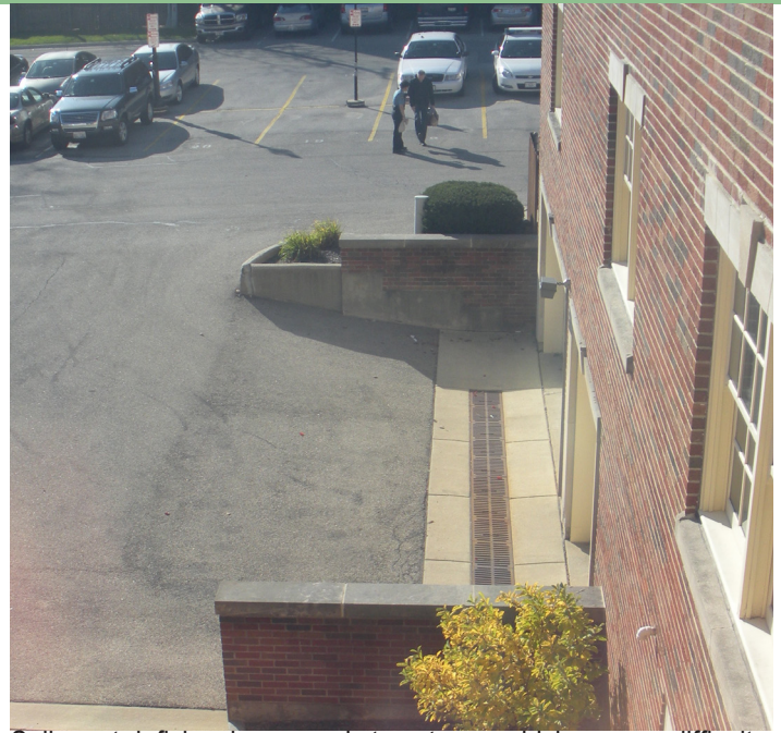
Sally port deficiencies: ramp is too steep, vehicle access difficult in bad weather, and backing out site lines are bad with site walls
