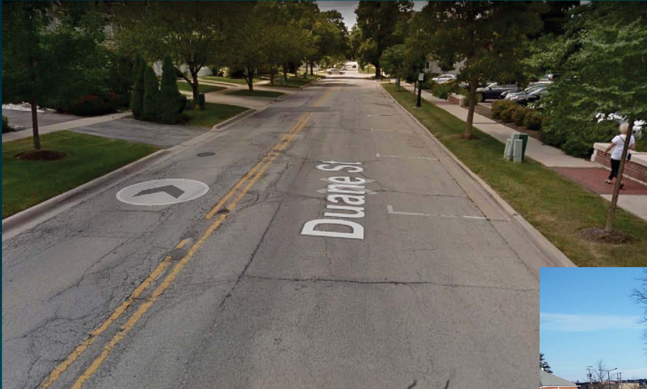
Current pavement condition
