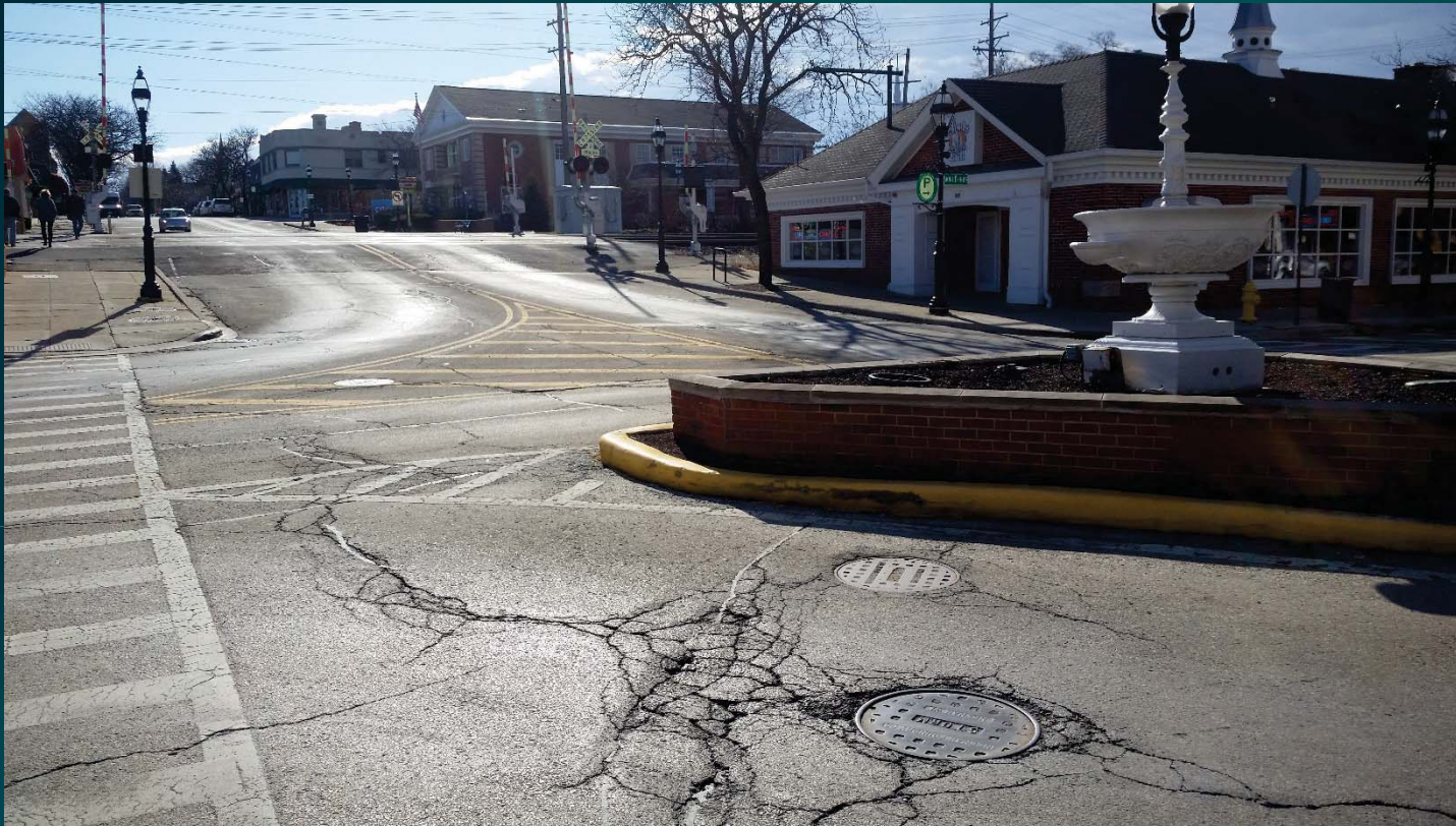
Current pavement condition
