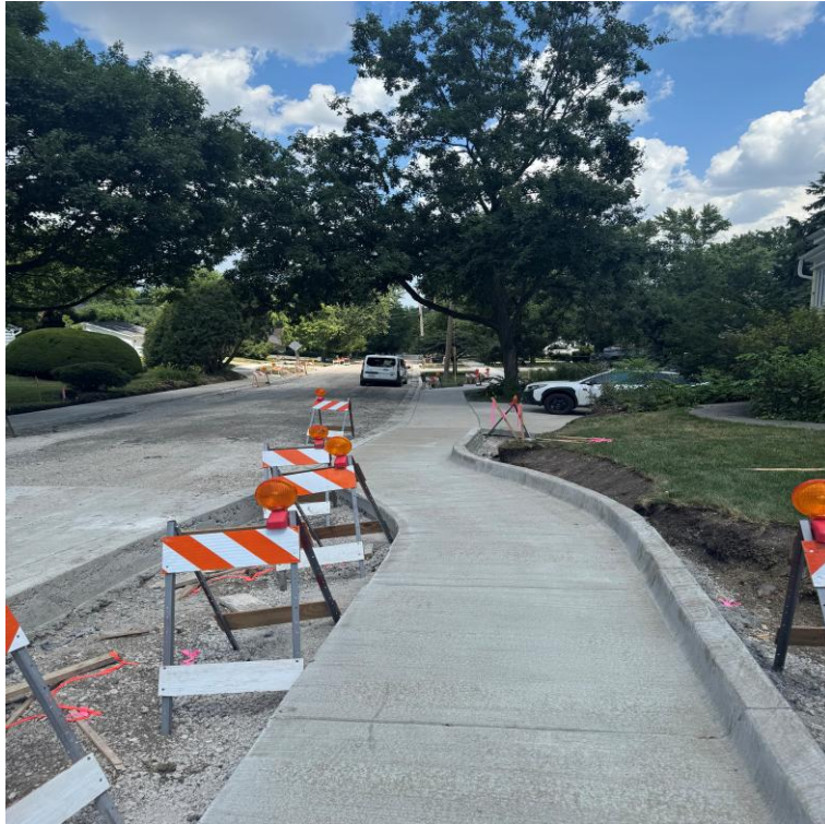
Newly constructed sidewalk on south side of Revere, just east of Bryant
