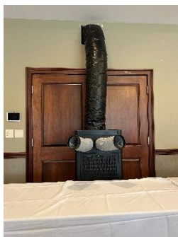
One of two temporary AC units brought in to help cool the Blue Heron Room due to failure of our HVAC RTU.
