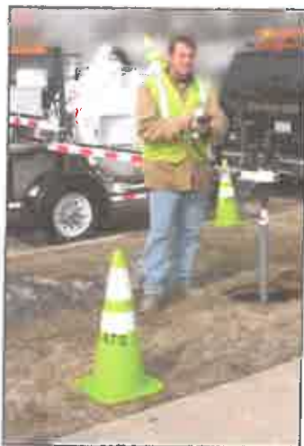
Computerized Valve Exercising and Assessment
