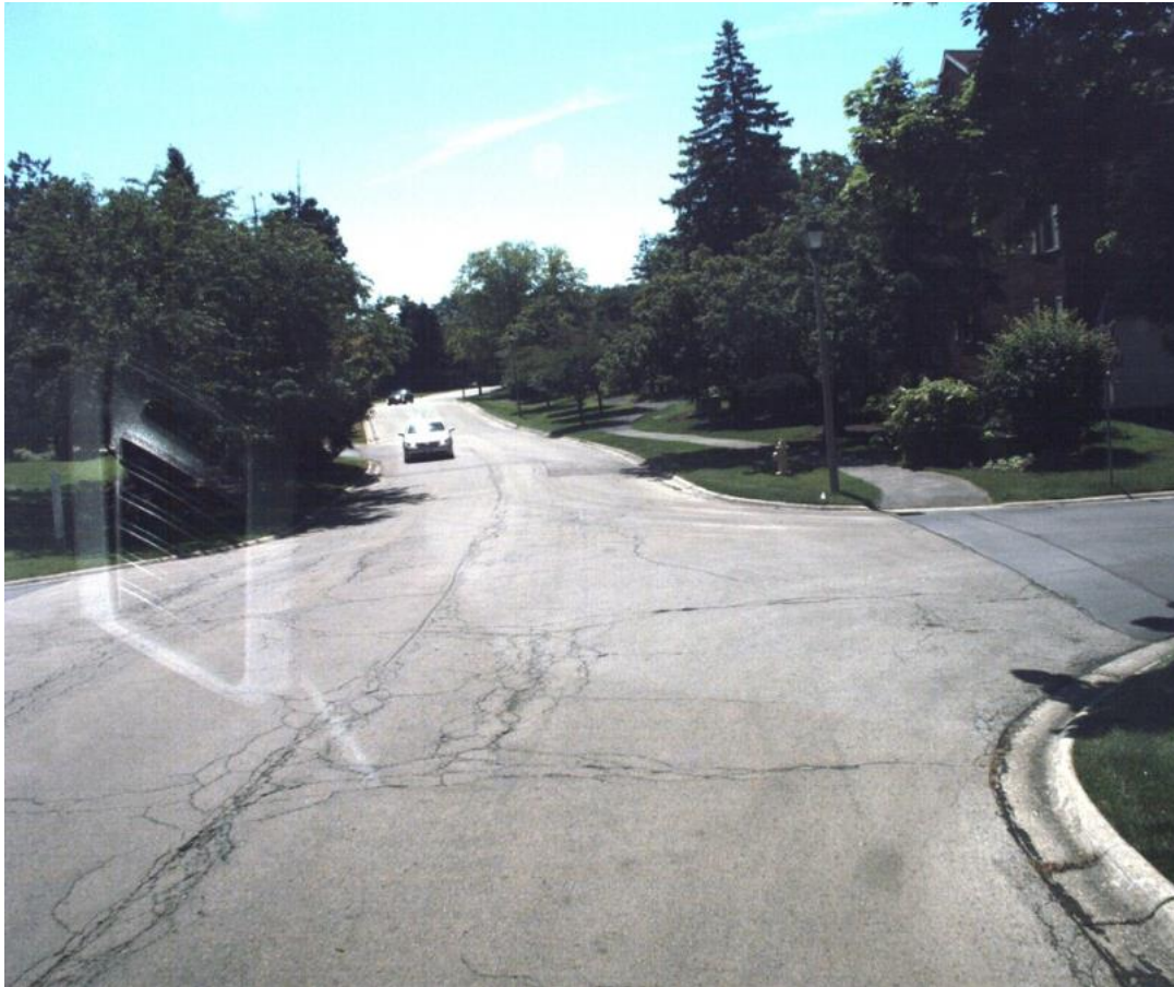
HILL AVE– Section 970 560 ft North of Acorn Ave to 460 ft South of Town Line PCI 17
