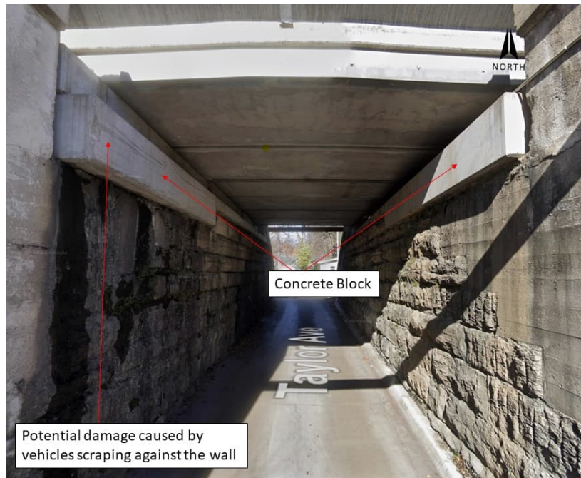
Figure 4. Potential Damage to Concrete Block
