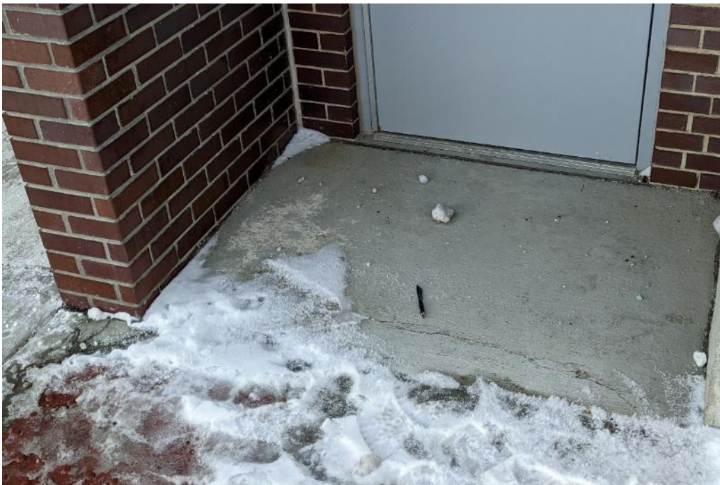
Photo 24. Concrete delaminated outside of west stair tower door at ground level.
