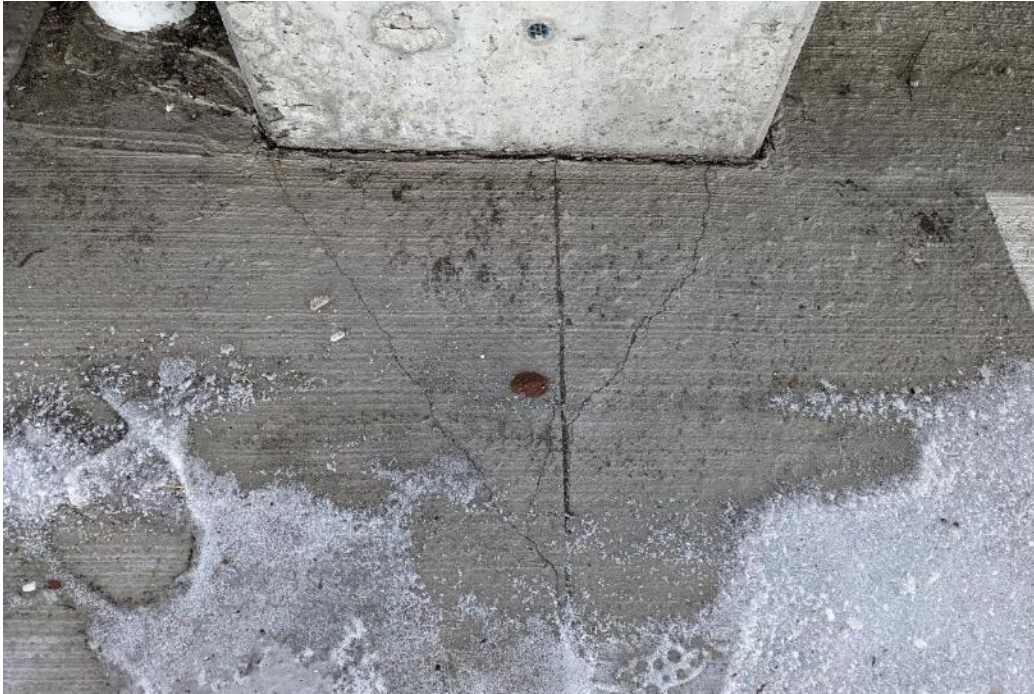
Photo 23. Typical diagonal slab-on-ground cracks off Finger columns.
