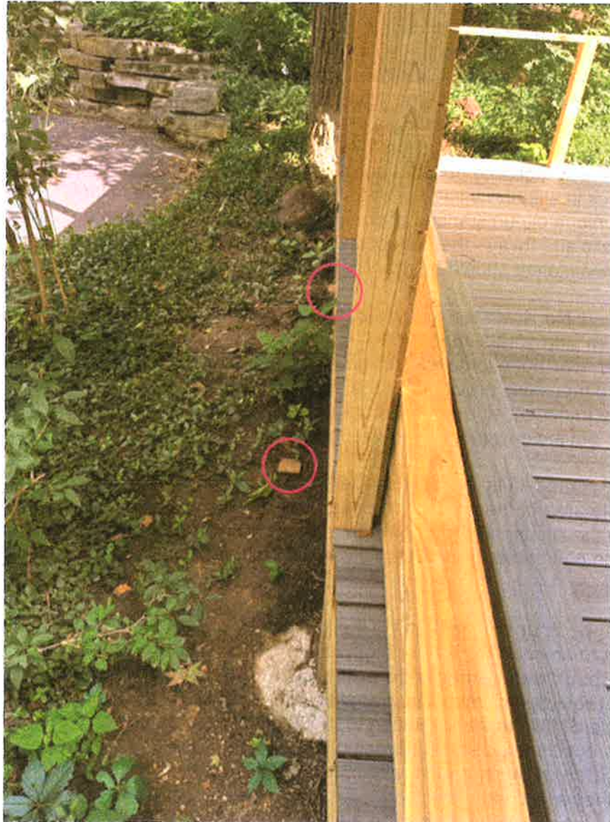
Figure 1. Former posts compared to new post to showcase new deck does not encroach onto neighboring property.
