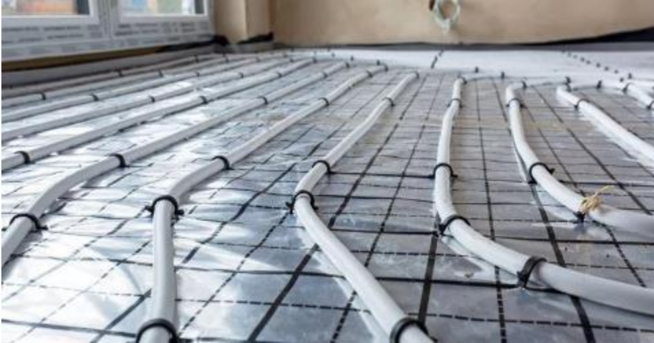
Hydronic floor heated System – glycol is circulated in the tubes.
