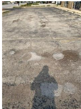
Front parking area, typical pavement condition for all three parking areas.
