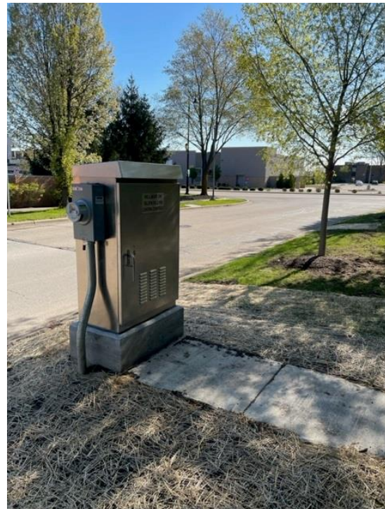
Street Light Controller with new ComEd Meter and Parkway Restoration
