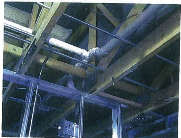
The new sewer system includes white PVC plastic vent pipes that run through the roof.
