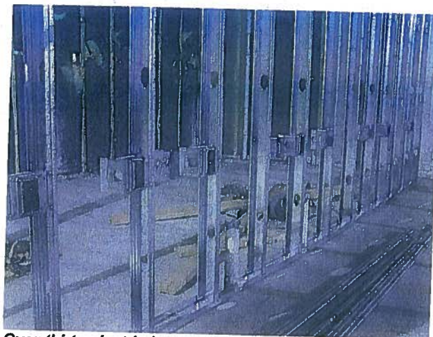
Over thirty electric boxes were installed in the kitchen. Many of these were on the main cooking line, above.
