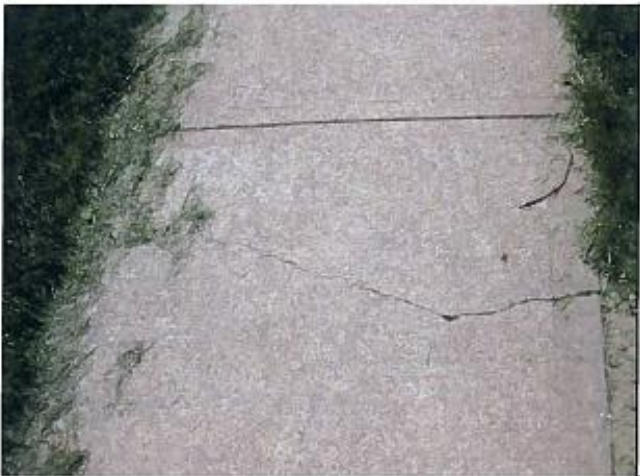
Figure 6N – Non-faulted Linear crack
