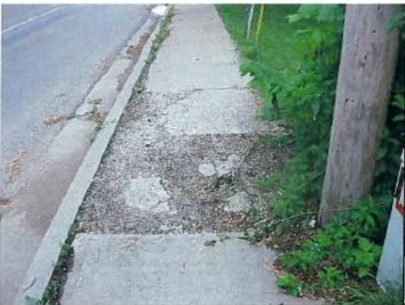
Figure 11H – High Severity Surface Defects
