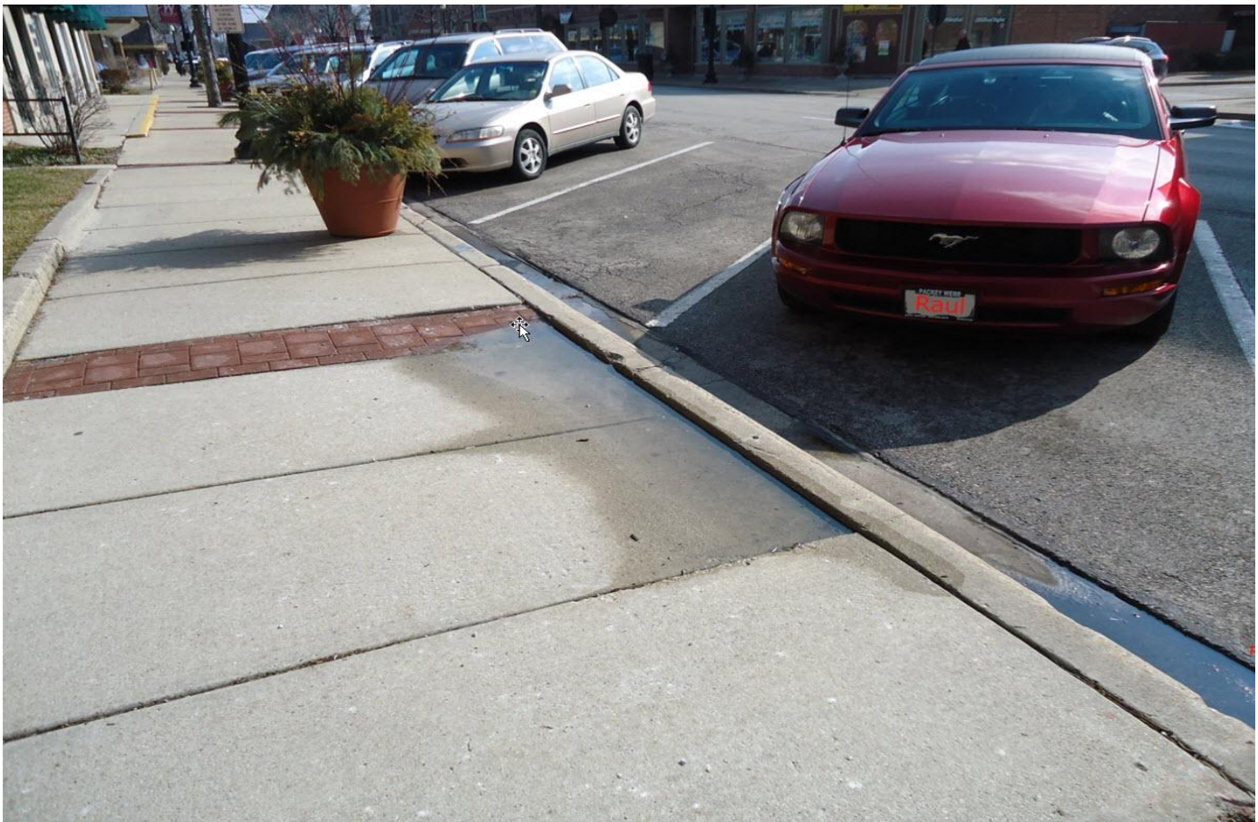
Figure 13 – Longitudinal Faulting Along Curbs
