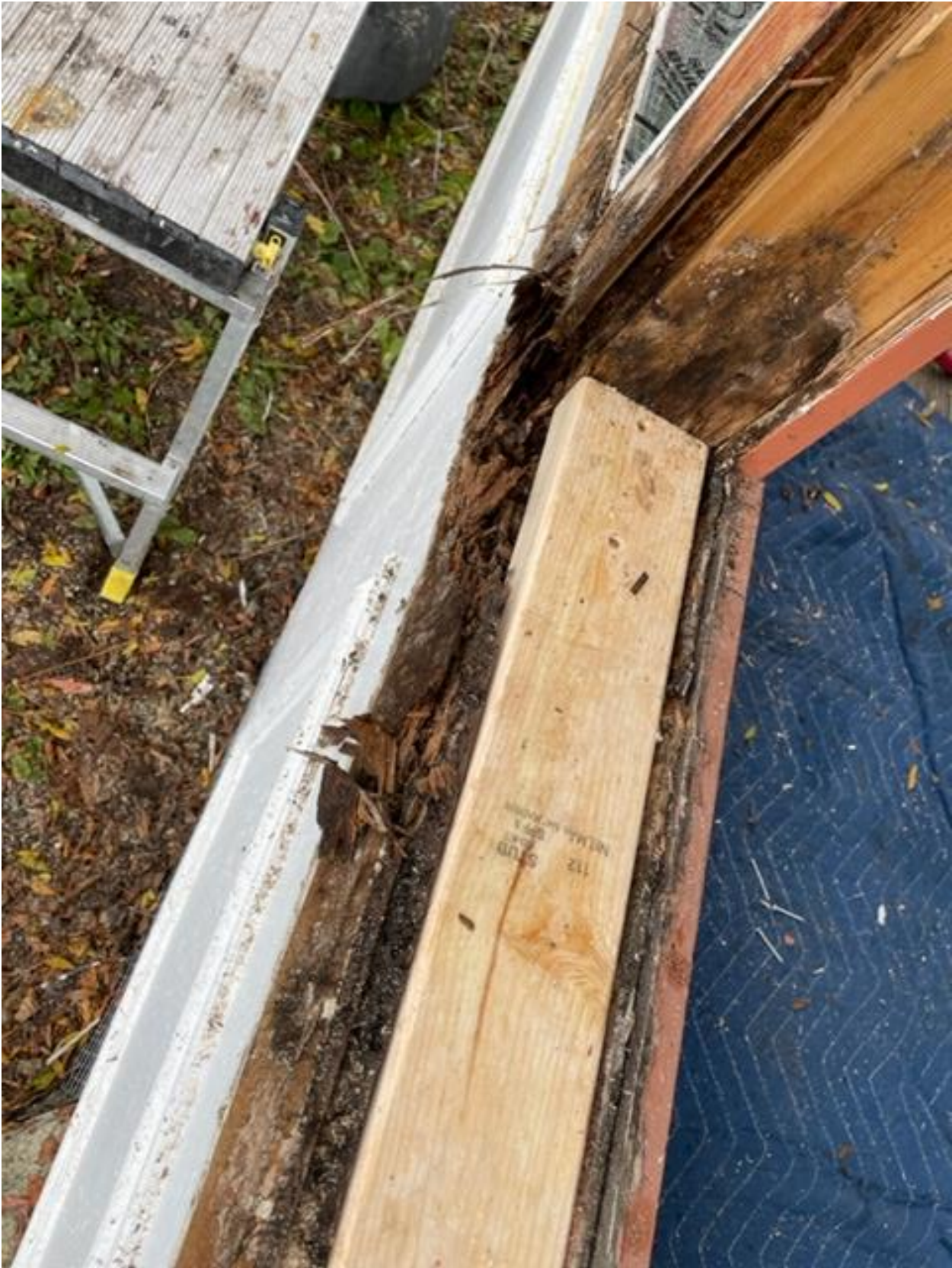
Wood rot on window casings
