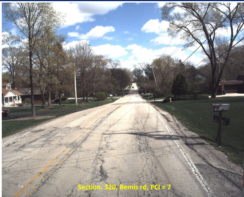
Figure 8: Sample pavement image with 'Failed' PCI value.
