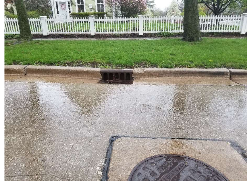
Failed adjustment ring(s) at 563 N Main St
