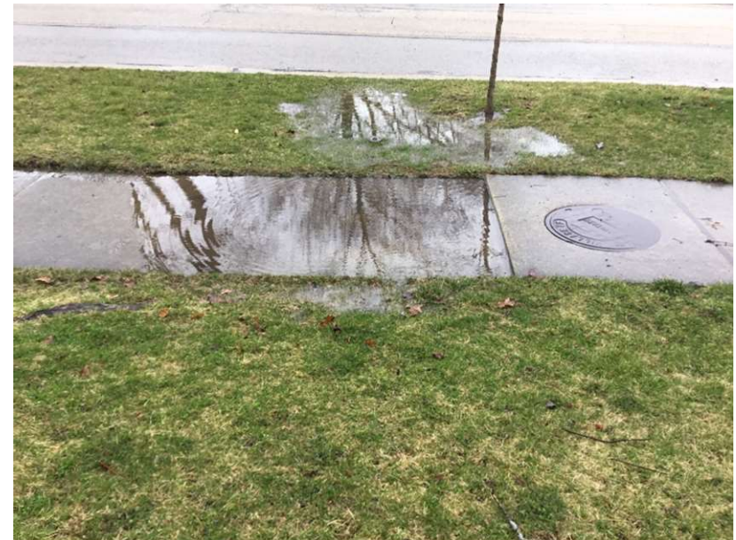
Sidewalk Drainage Issue at 150 N Kenilworth Ave
