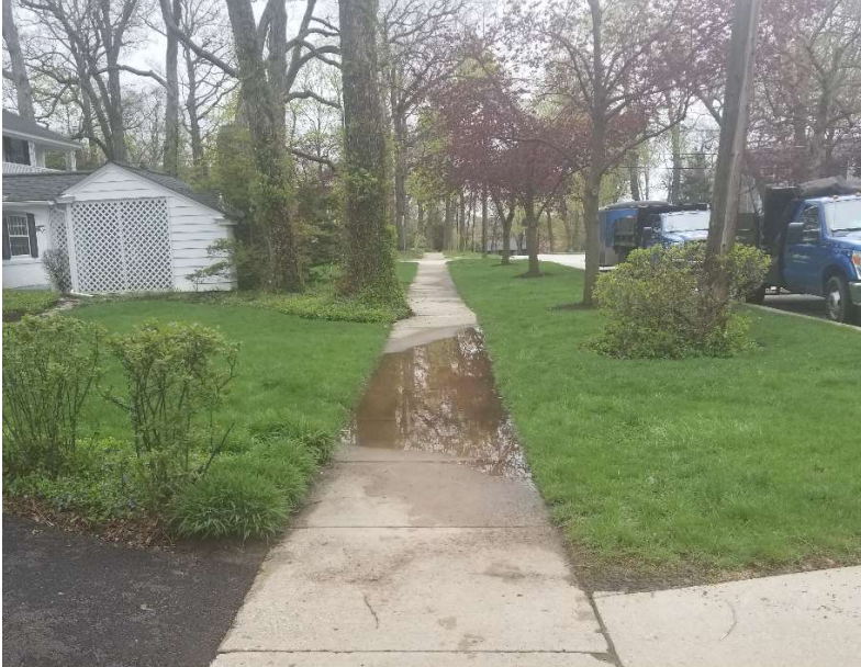
Sidewalk Drainage Issue at 706 Forest Ave (request from resident)
