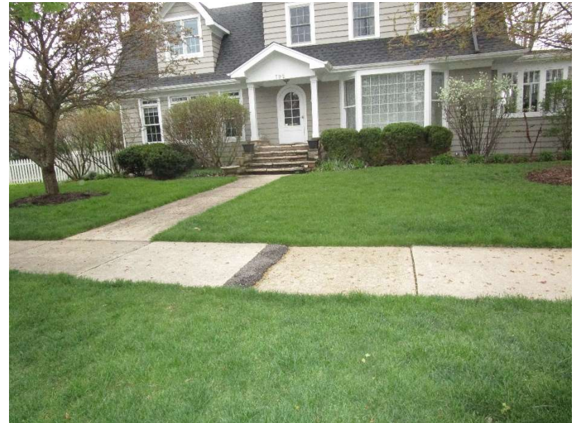
Sidewalk Displacement at 792 Forest Ave
