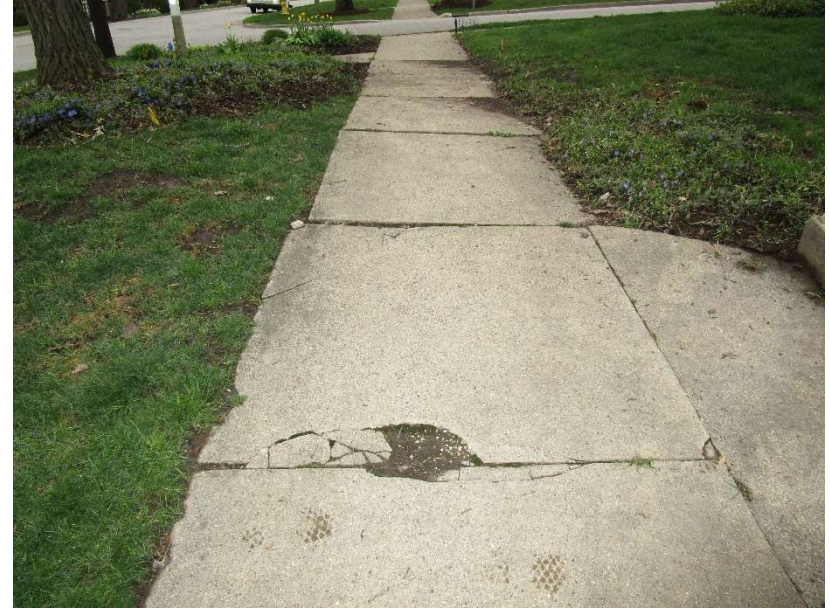
Broken Sidewalk at 710 N Park Blvd
