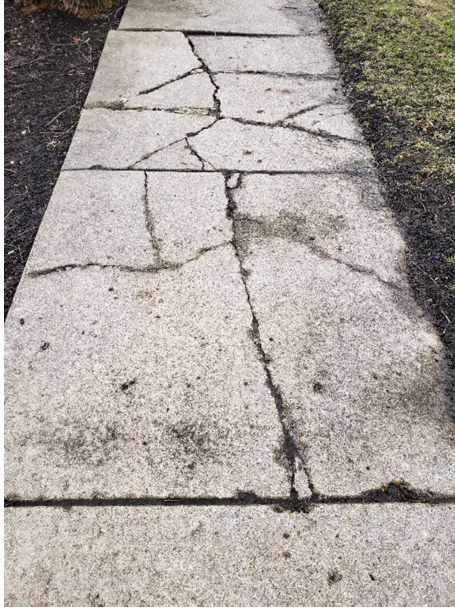
Broken Sidewalk at 45 S Park Blvd (request from resident)
