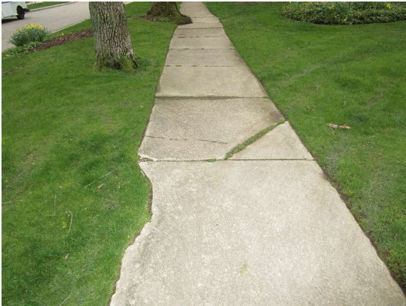
Broken Sidewalk at 606 Forest Ave
