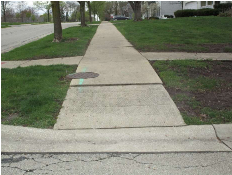
Sidewalk Displacement and Noncompliant Ramp at 772 Fairview Ave
