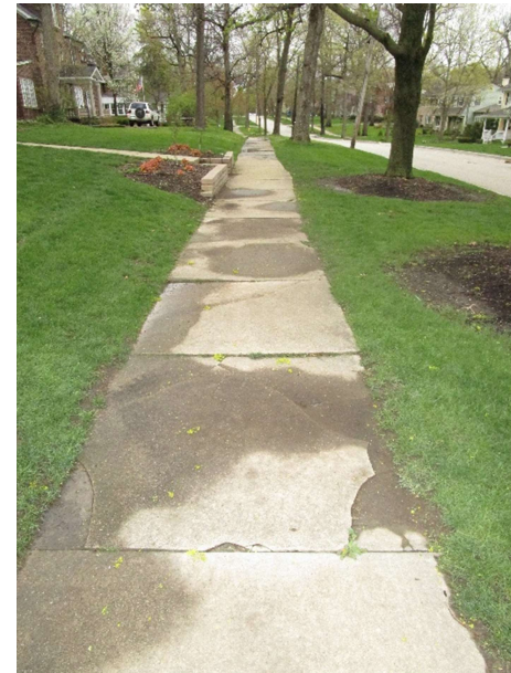
Broken Sidewalk at 656 Forest Ave
