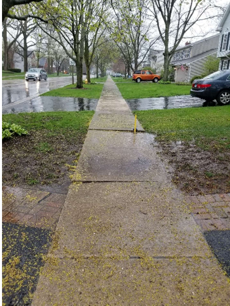
Sidewalk Displacement at 762 Glenbard Rd (request from resident)
