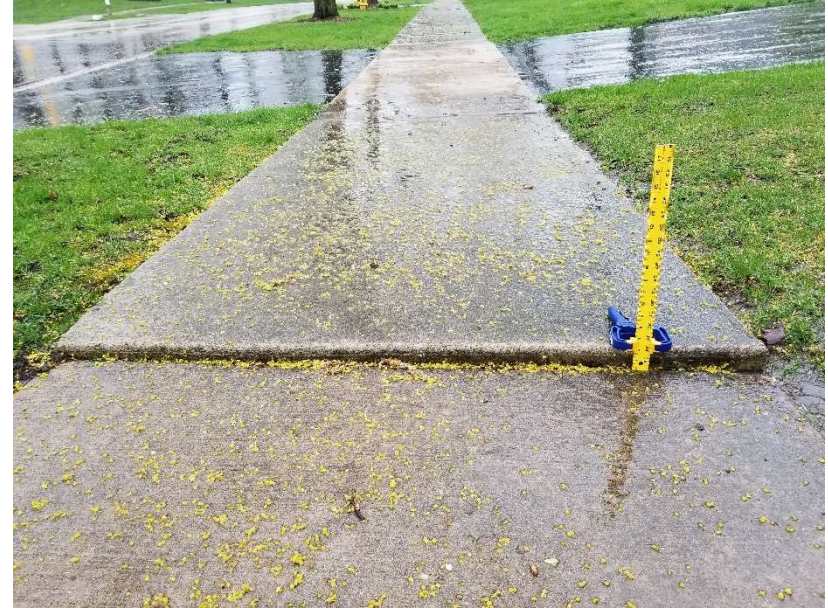
Close-up of Sidewalk Displacement (~1 3/4") at 762 Glenbard Rd
