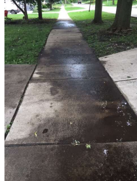
Sidewalk Drainage Issue at 297 Bryant Ave (request & photo from resident)
