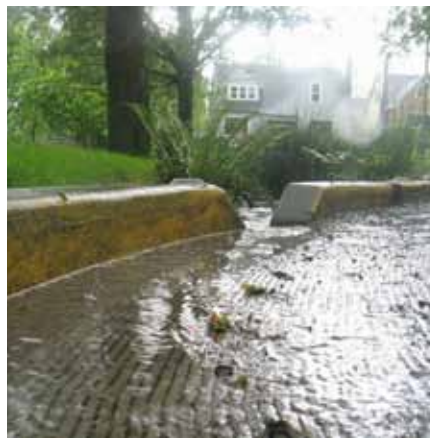
Curb inlet that allows stormwater to flow directly into infiltration basins or rain gardens
