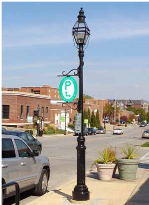
Existing gas lamp light standard
