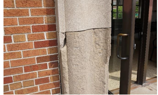
Masonry damage at platform to station entry
