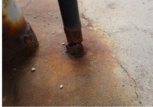
Aging Infrastructure and Structure
