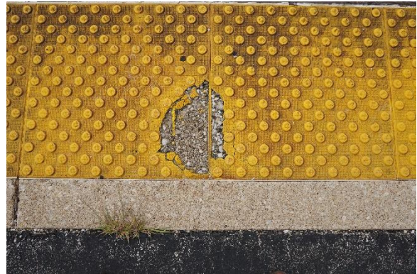
Figure 11: Damaged tactile warning strip at platform edge
