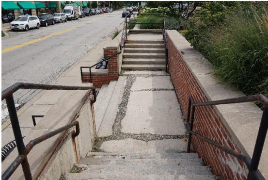
North retaining wall, stairs, and handrail showing cracking, and deterioration
