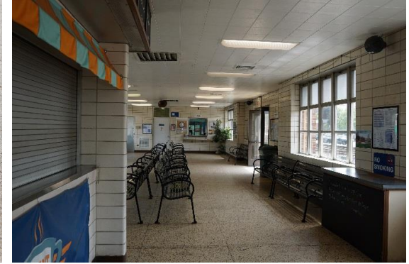
Waiting room is undersized, limited heating and ventilation
