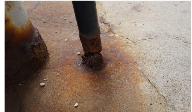
Rusted Lally Column (L), Rusted through leader (R)
