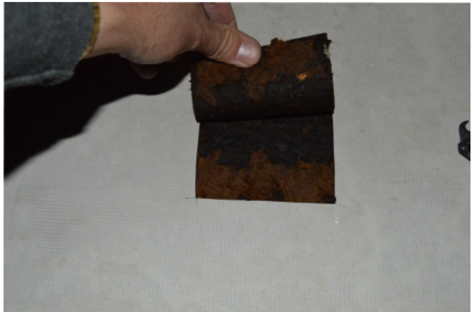
Core sample taken at location 3. Note the darker-colored wood fiber recovery board that is completely saturated with moisture
