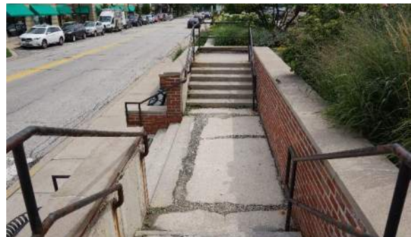
Figure 10: North retaining wall, stairs, and handrail showing cracking, and deterioration
