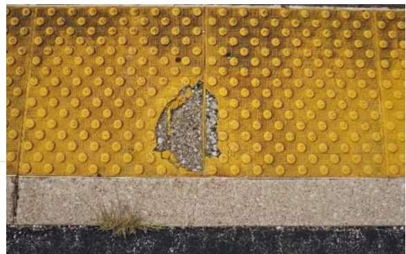
Figure 11: Damaged tactile warning strip at platform edge
