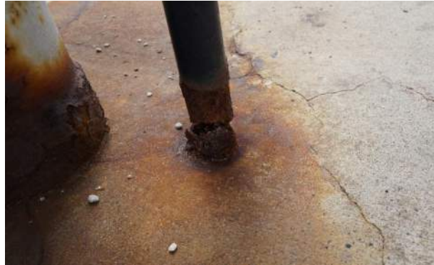
Figure 9: Rusty Lally Column (L), Rusty through leader (R)
