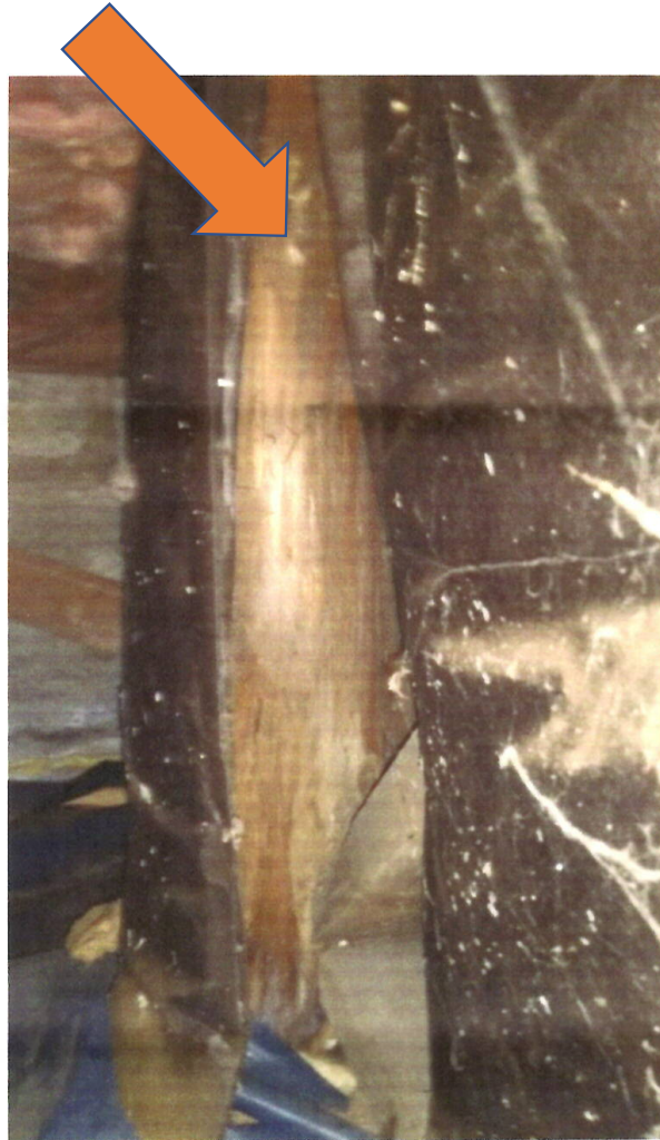
Picture of tree stump in crawl space supporting an addition
