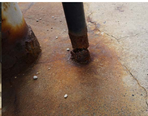
Rusting concrete column and drainage Pipe
