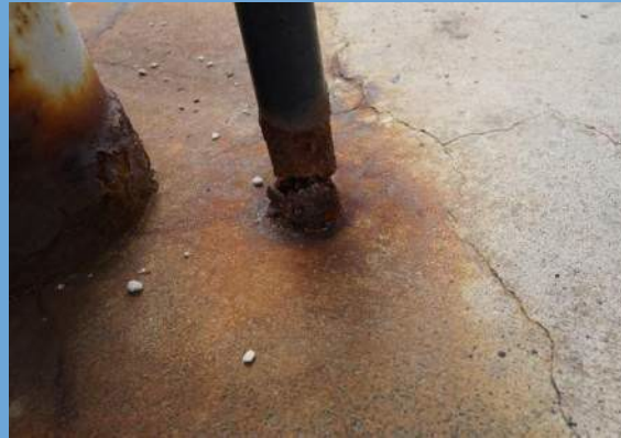
Aging Infrastructure and Structure
