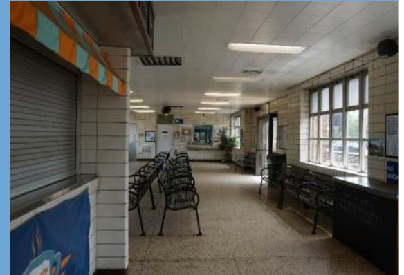
Waiting room is undersized, limited heating and ventilation
