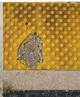
Cracked Tactile Warnings along platform edge
