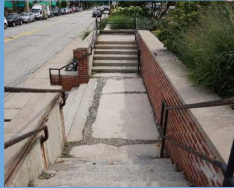
Stairs and Masonry-Aging
