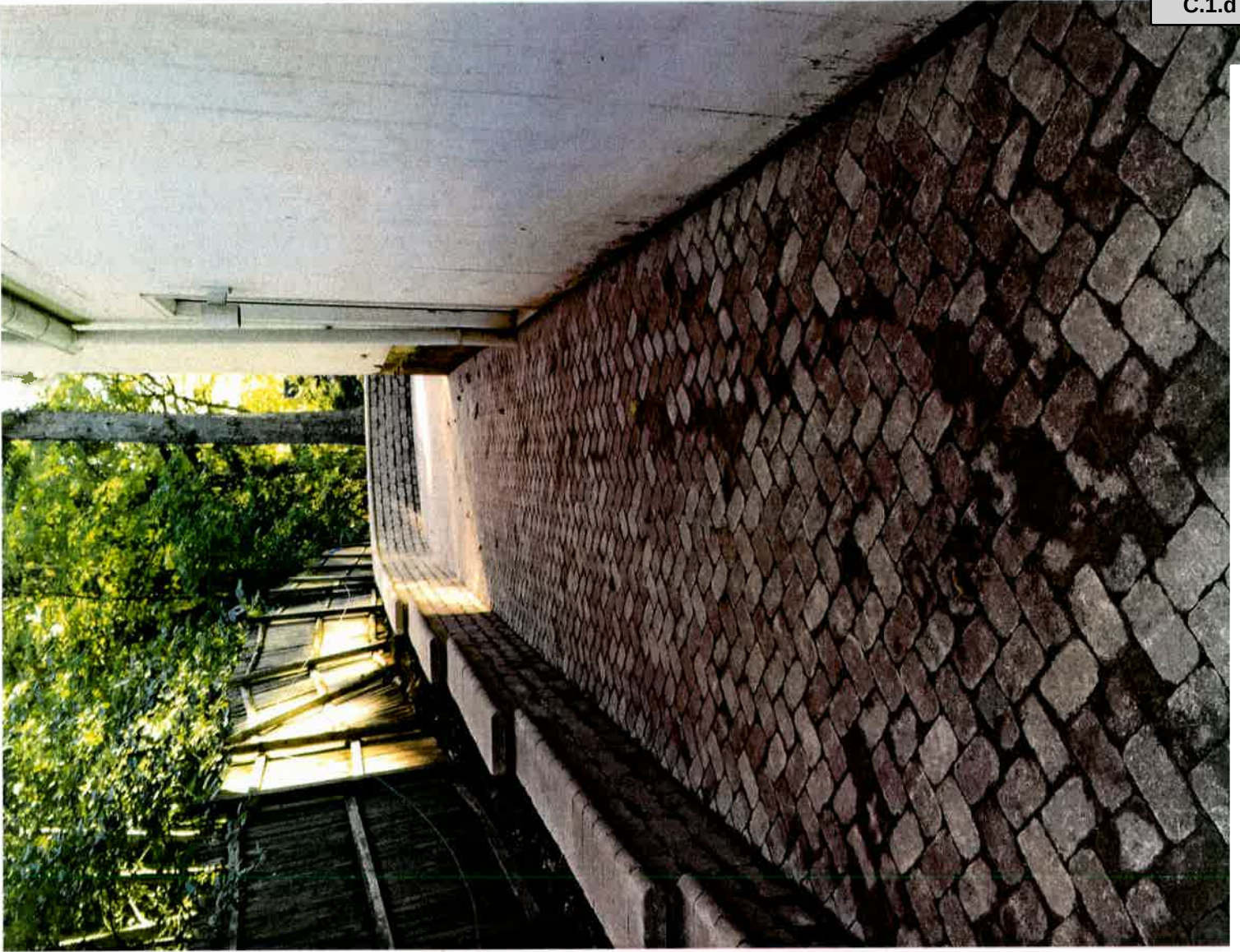
Attachment: Photos - Existing Conditions (3782 : 787 Crescent Blvd. - Accessory Structure Setback & Impervious Surface Setback - CNV)
