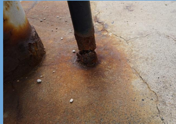
Aging Infrastructure and Structure
